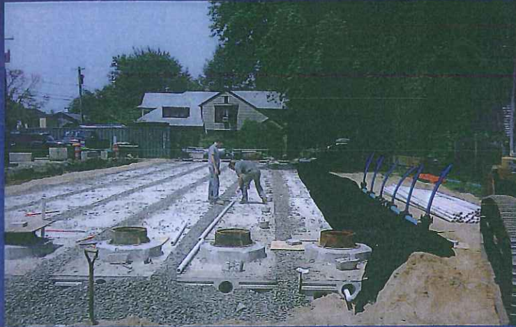
Large Scale Subsurface Wastewater Absorption System Construction - Leaching Galleries and Access Manholes
